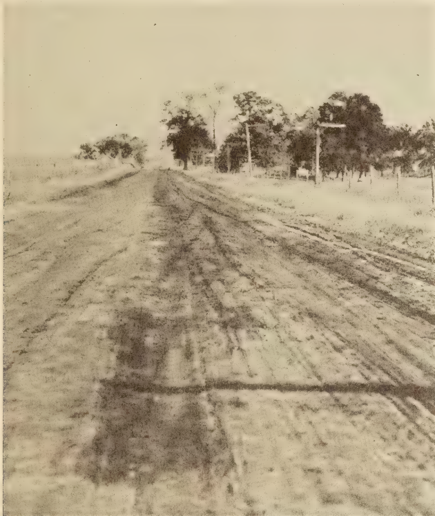
FIGURE 4.—POORLY DRAINED SECTION. THE IRREGULAR SURFACE HAS CAUSED TRAFFIC TO FOLLOW SELECTIVE TRAFFIC LANES. AS A RESULT PORTIONS OF THE SURFACE HAVE BEEN DEPRIVED OF THE IRONING AND KNEEDING EFFECT OF TRAFFIC AND HAVE RAVELED EXTENSIVELY
